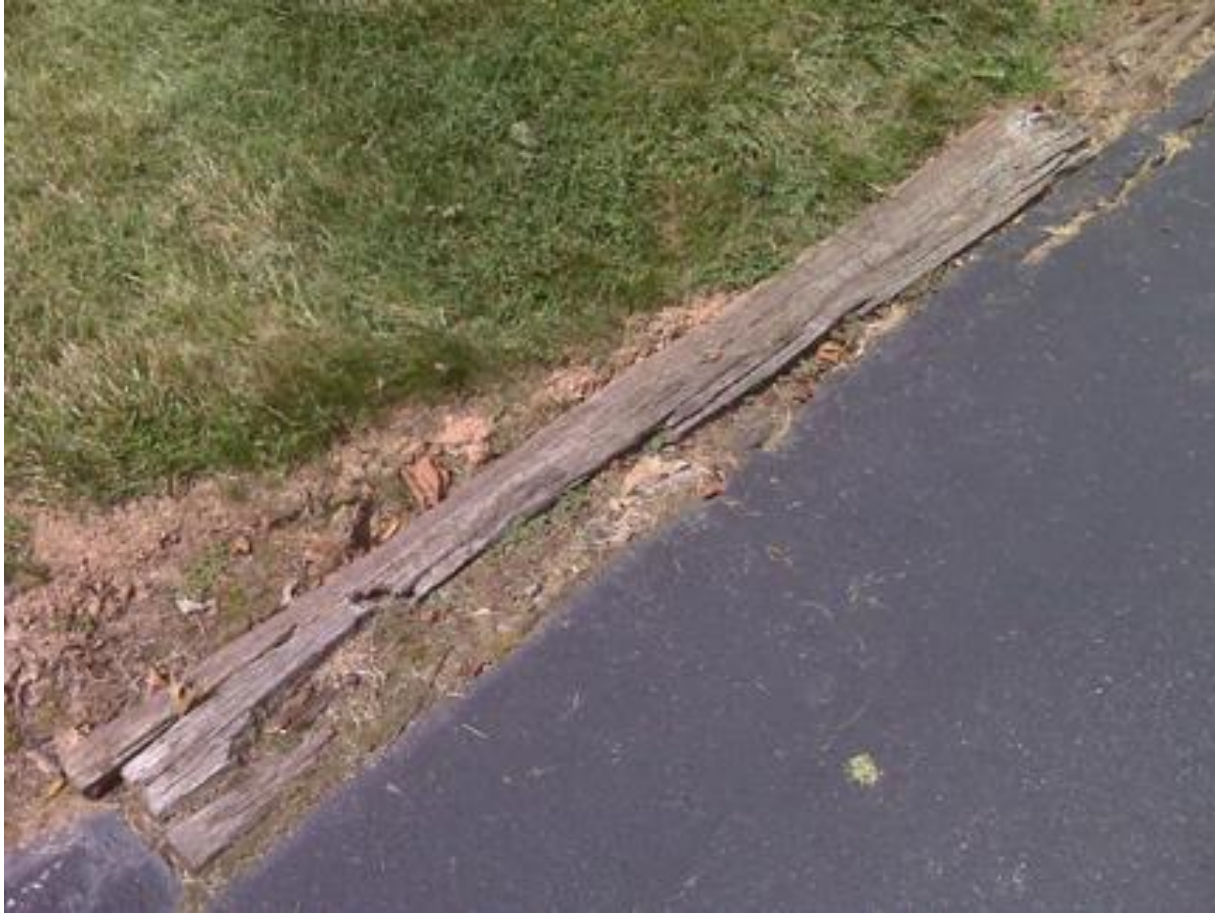
Figure 8.3 Curb in Very Poor Condition
