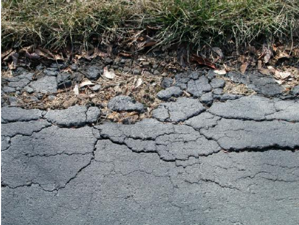
Figure 7.3 Driveway in Poor Condition
