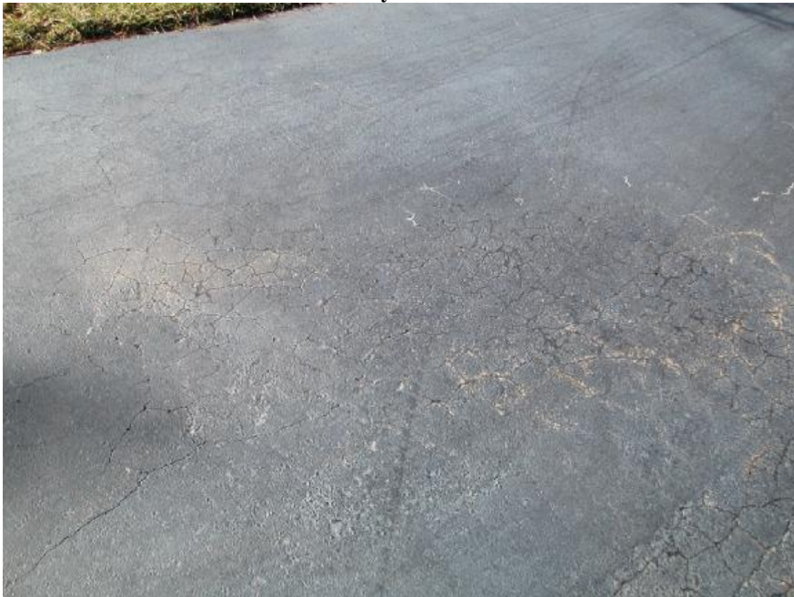
Figure 7.2 Driveway in Poor Condition
